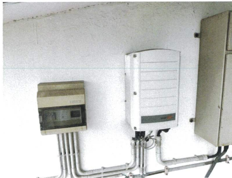
Photovoltaic cells control unit
