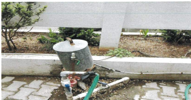
Bore well inside the Campus
